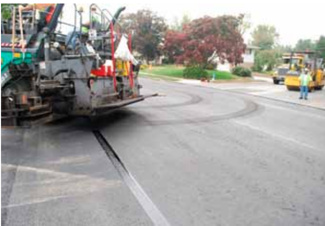
The paver turns on the paving fabric without damaging the fabric. Loader tri-axle trucks also traveled across the fabric with no resulting damage. Photo courtesy of ISMF LLC.
