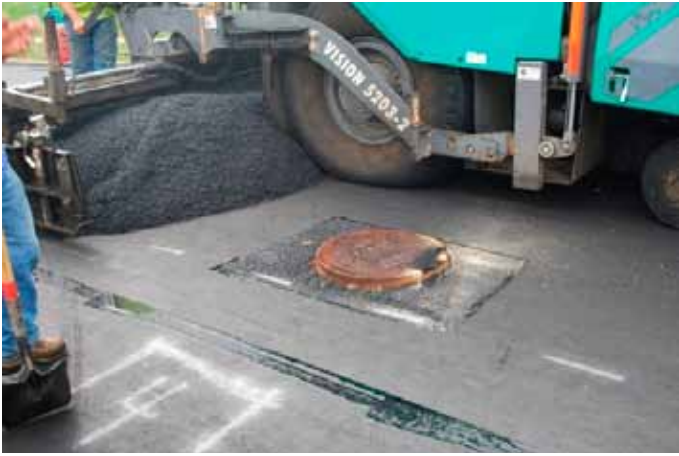
The paving fabric is placed around a sanitary sewer manhole. PG 64-22 material was used to seal the fabric overlap. Photo courtesy of ISMF LLC.
